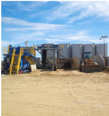
We installed the modular processing solution at Anadarko's strip site in just 20 days.
