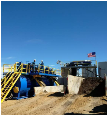
Jared Brady and Adam Kesterholt of Newalta work on the site's receiving tank.
