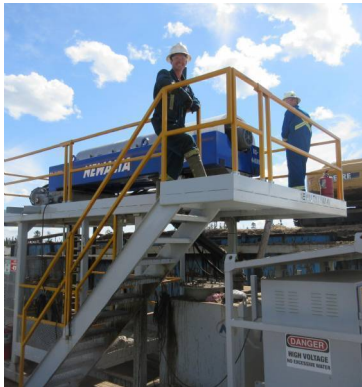
Onsite technicians monitor solids consistency for dryness and adjust centrifuge parameters accordingly.
