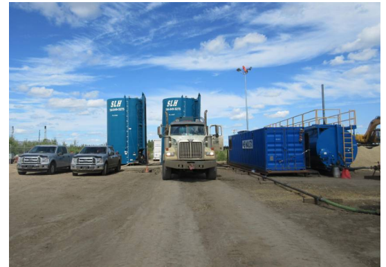
Trucks from surrounding producer sites deliver slop volumes to feed tanks for consolidation prior to processing activity.
